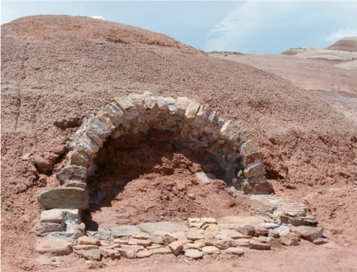
Figure 7 The first three arches of a vault completed at the end of Crew 22's rotation.
