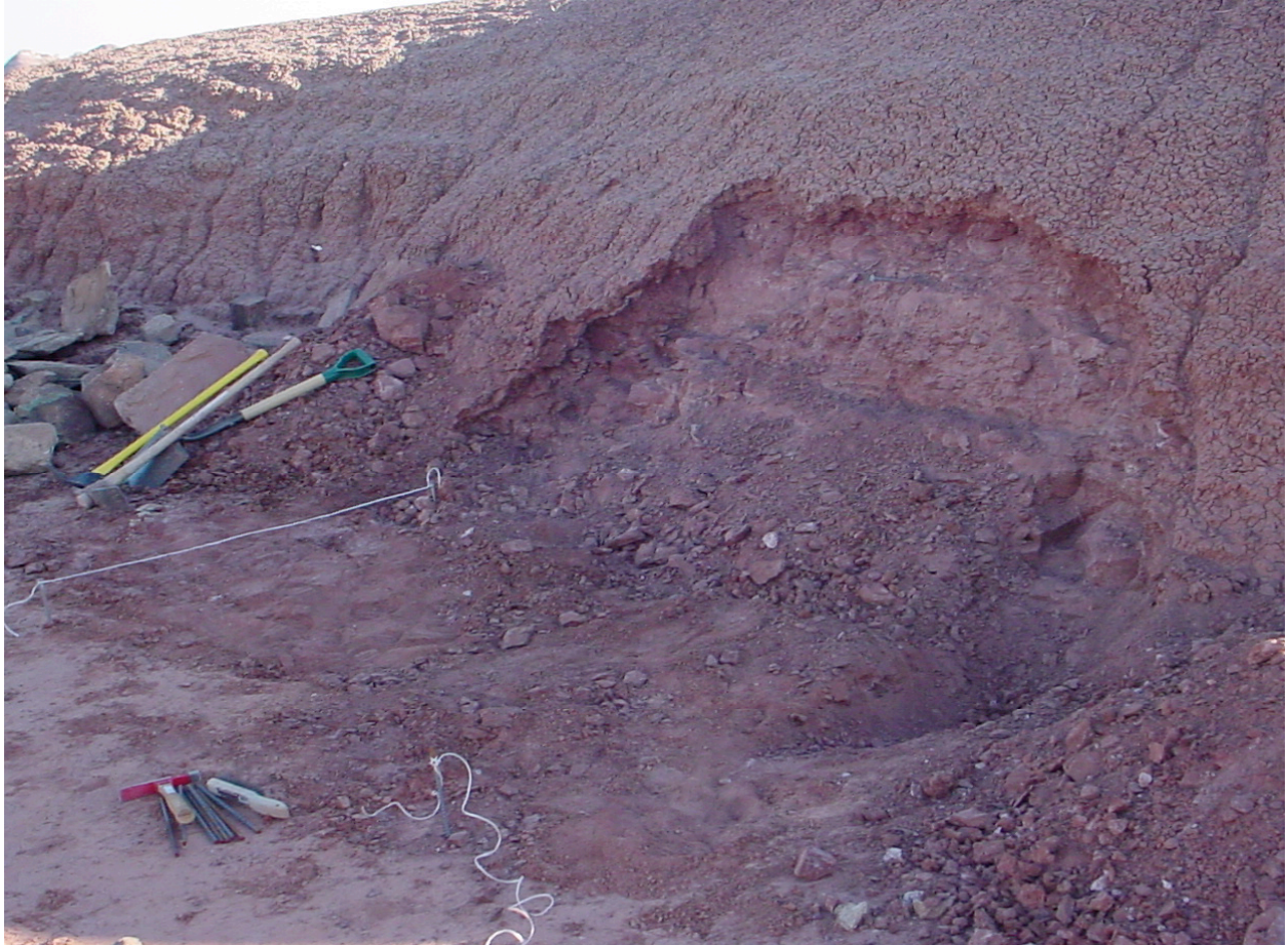
Figure 2 Excavation of the top crumbly layer exposes relatively solid rock on which the vault was constructed.
